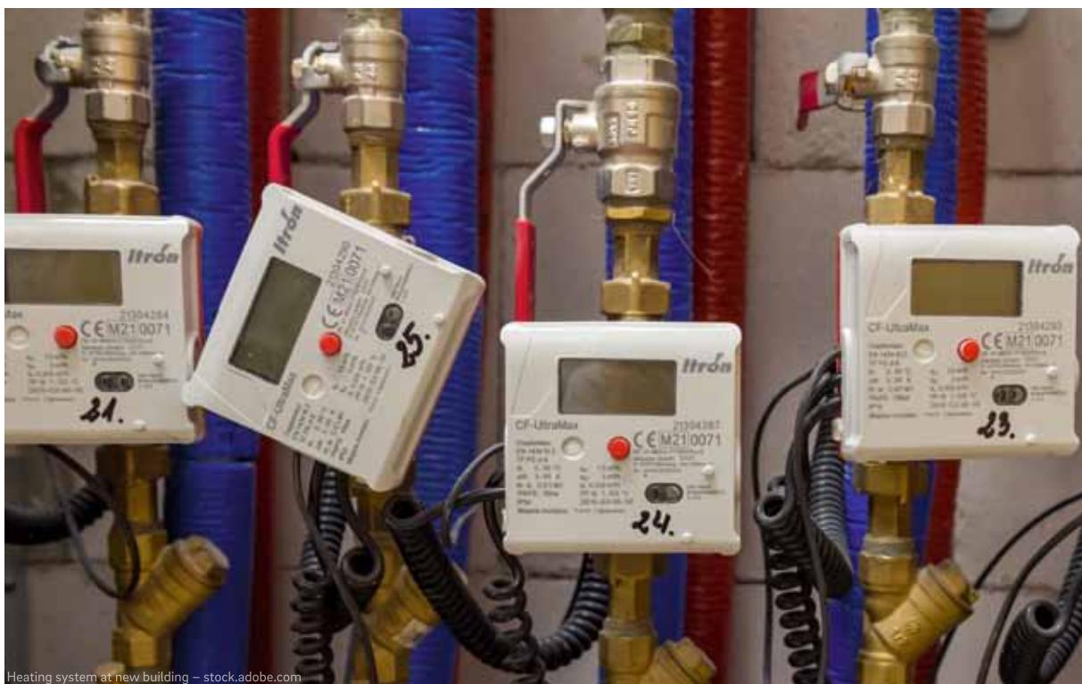
Heating system at new building – stock.adobe.com
